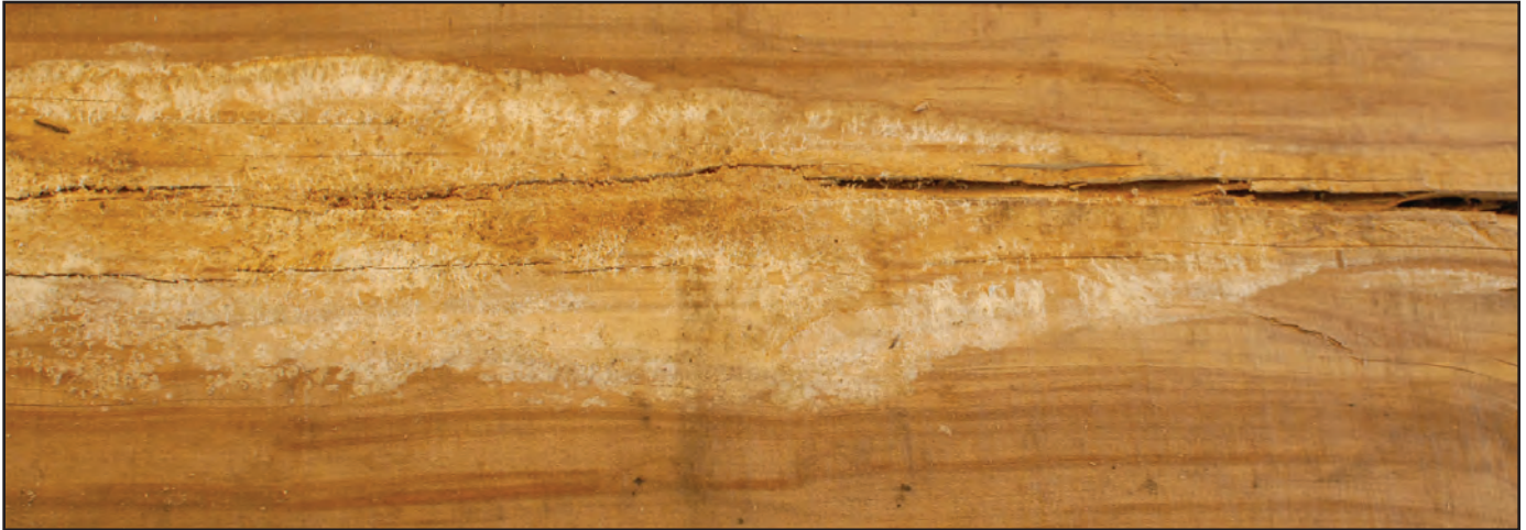
Figure 2. Incipient decay ("stack burn") in a sweet gum tie.
