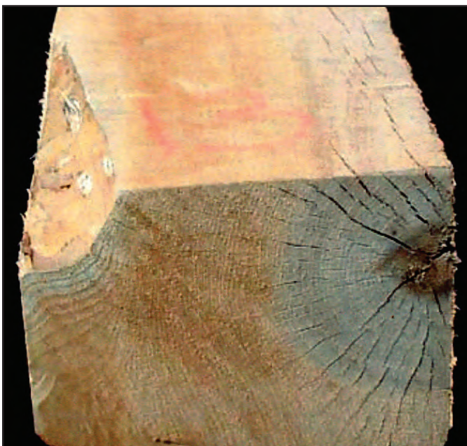
Figure 15. Wane outside the rail-bearing area. Would this be acceptable?
