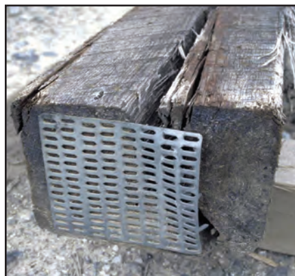
Figure 30. End plates can't salvage every tie.
