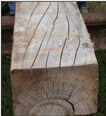
Figure 37. Since sweet gum normally has interlocking grain, the evident slope of grain in this tie would be acceptable. Figure 3 showed a good example of a sweet gum tie with interlocking grain, so it's repeated here. The shake would have to be looked at too.
