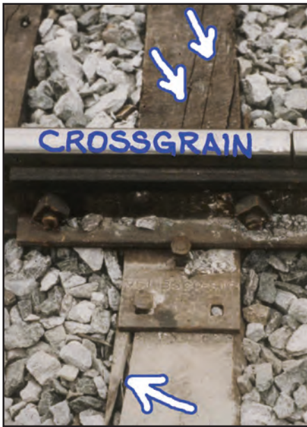
Figure 35. Crossgrain in this tie caused it to fail prematurely.
