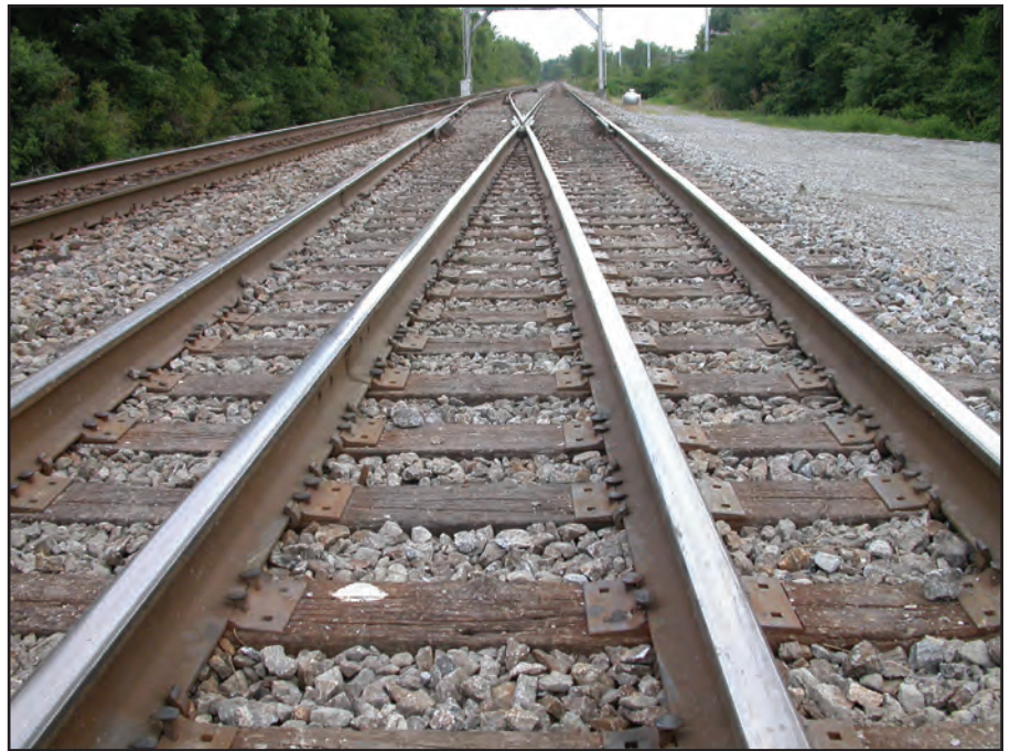
Figure 11. The use of switch ties, where two sections of track are joined by one long wooden tie.
