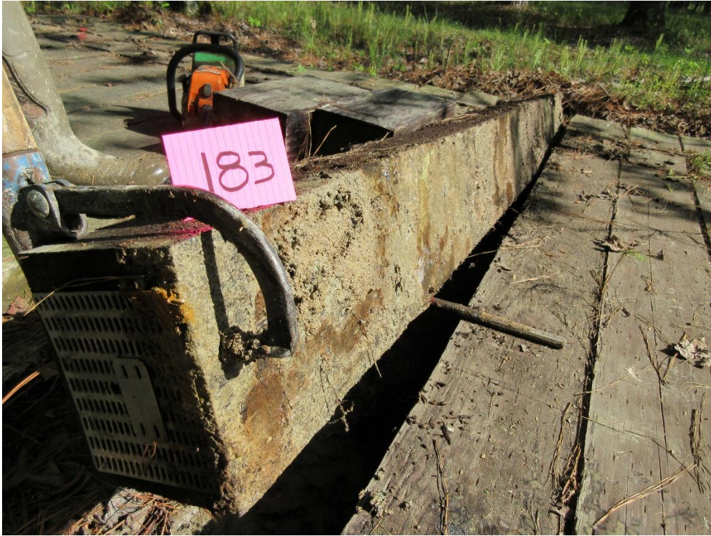
Figure 39 – Tie #183 Douglas fir/P2 creosote (Lonza).
