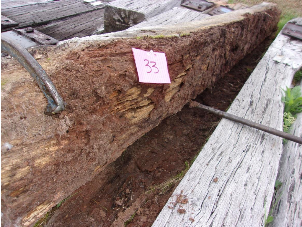
Figure 59 – Tie #33 untreated white oak with decay and termite damage.
