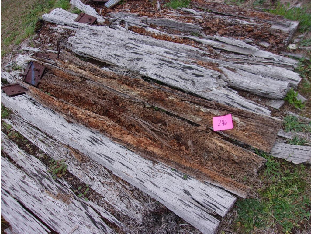
Figure 103 – Tie #246 untreated red oak with failed due to decay and Formosan termites.
