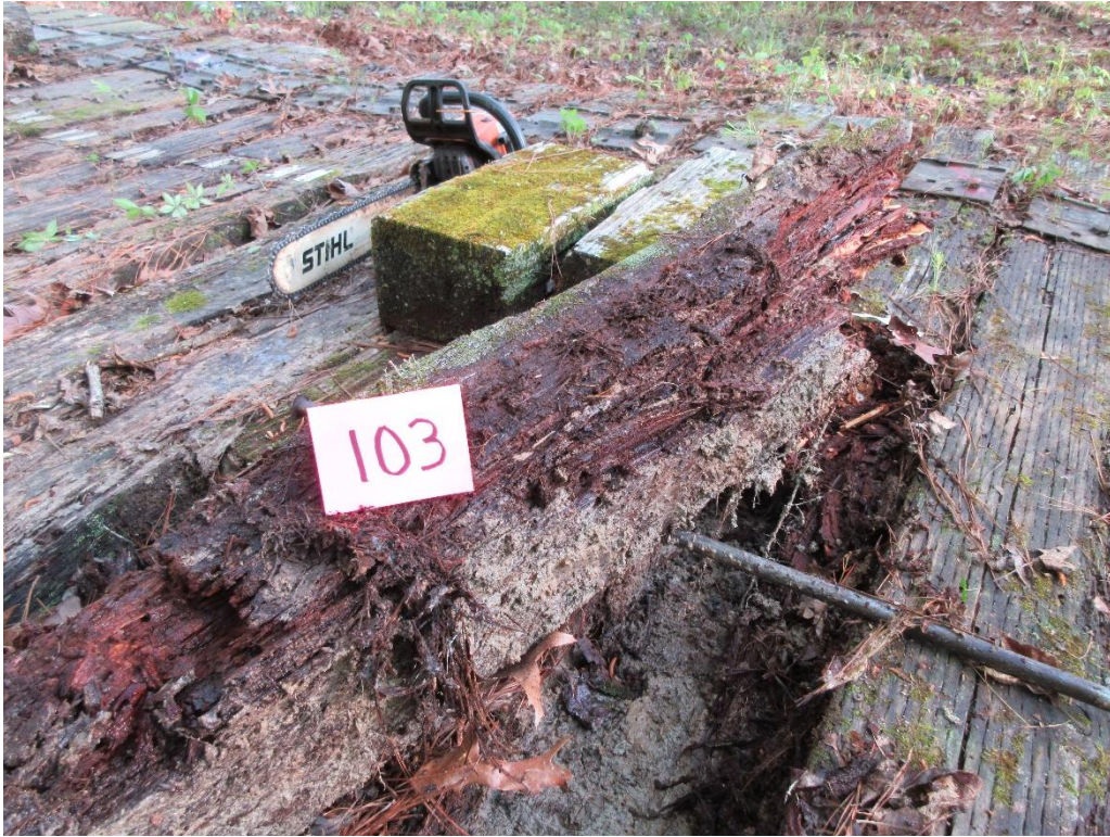
Figure 21 – Tie #103 untreated Douglas fir which failed due to decay.
