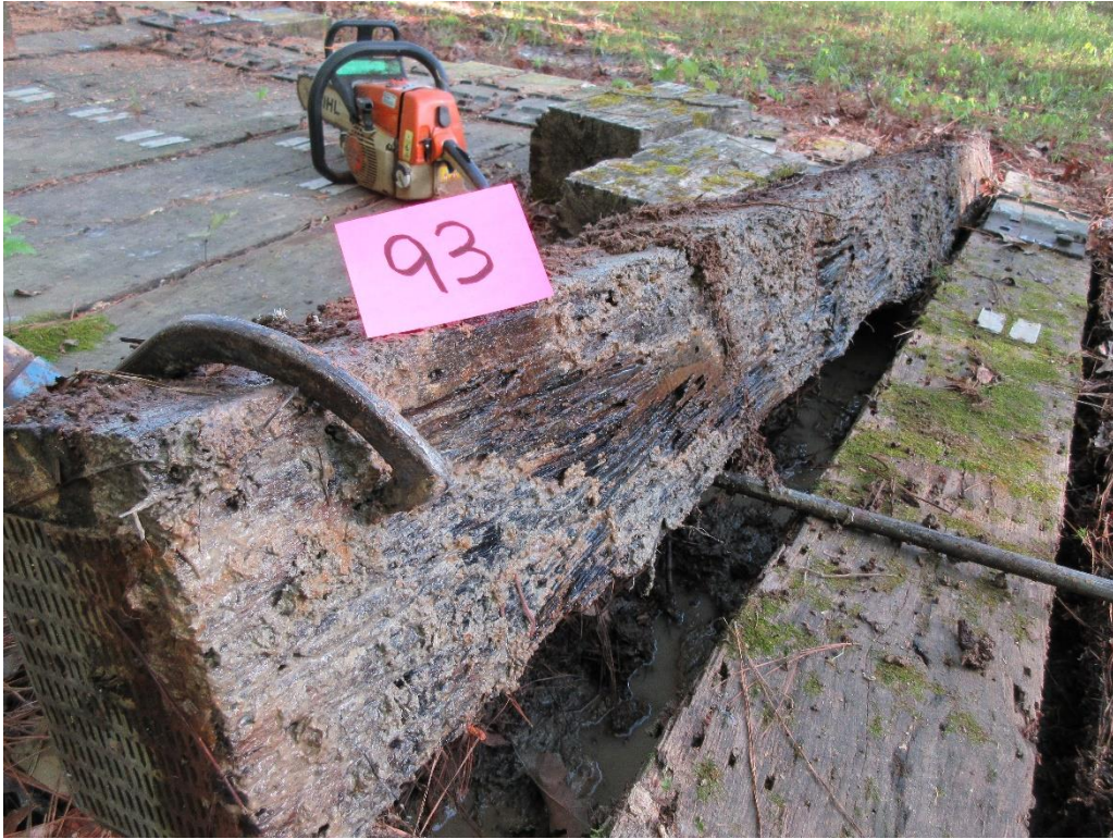
Figure 19 – Tie # 93 untreated white oak width moderate decay and termite damage.
