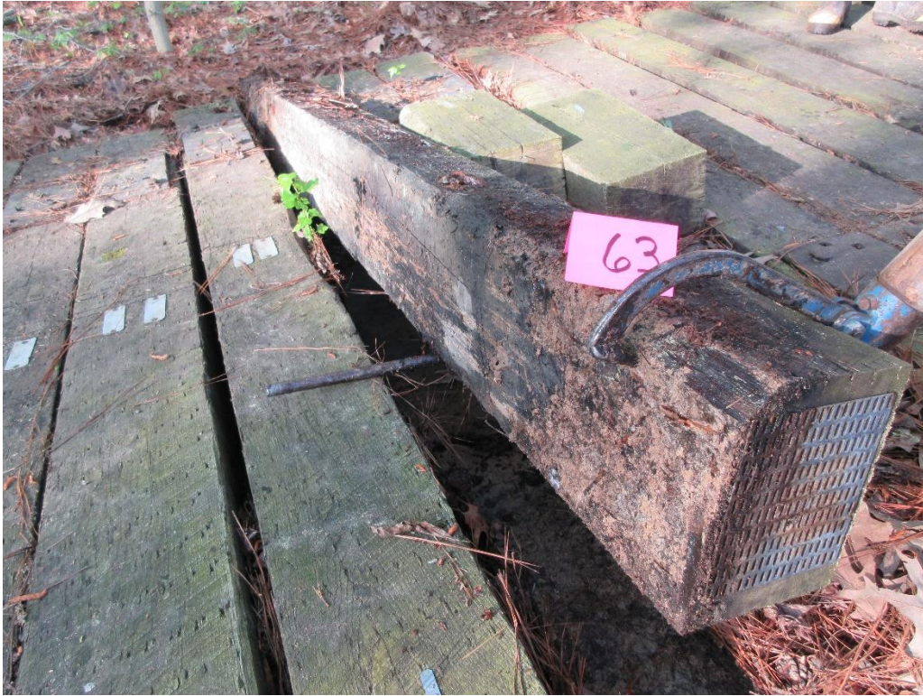
Figure 13 - Tie #63 red oak/1 step creosote borate with trace decay (Stella Jones).
