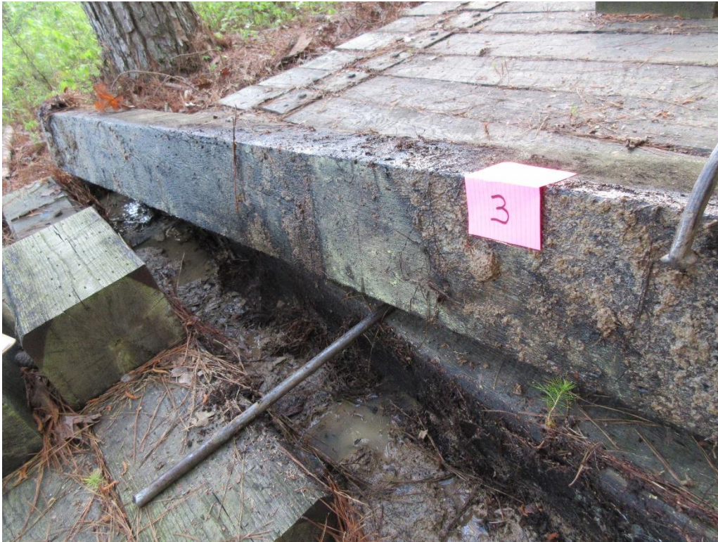
Figure 1 - Tie #3 white oak/borate/creosote 6# (Koppers).
