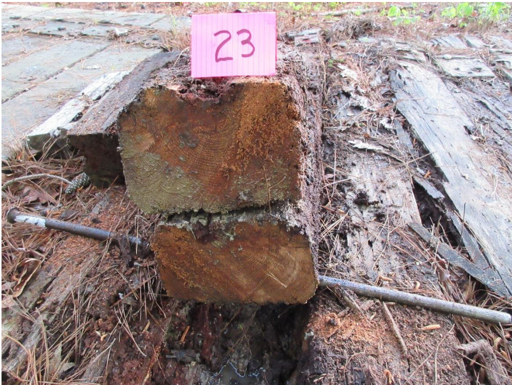
Figure 6 – Tie #23 untreated red oak with extensive decay and moderate termite damage.
