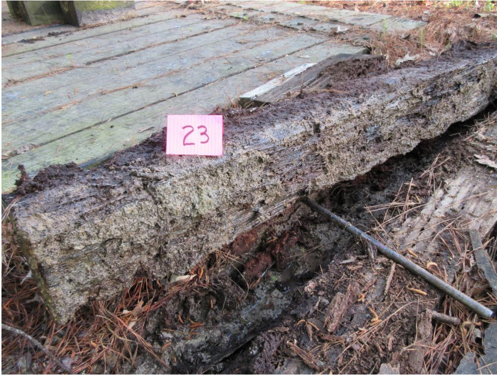
Figure 5 – Tie #23 untreated red oak with heavy decay and moderate termite damage.
