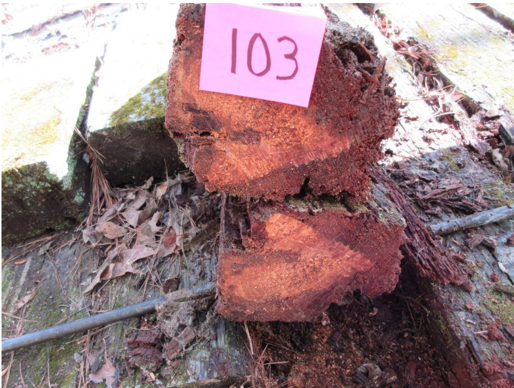
Figure 22 - Tie #103 severely decayed untreated Douglas fir.
