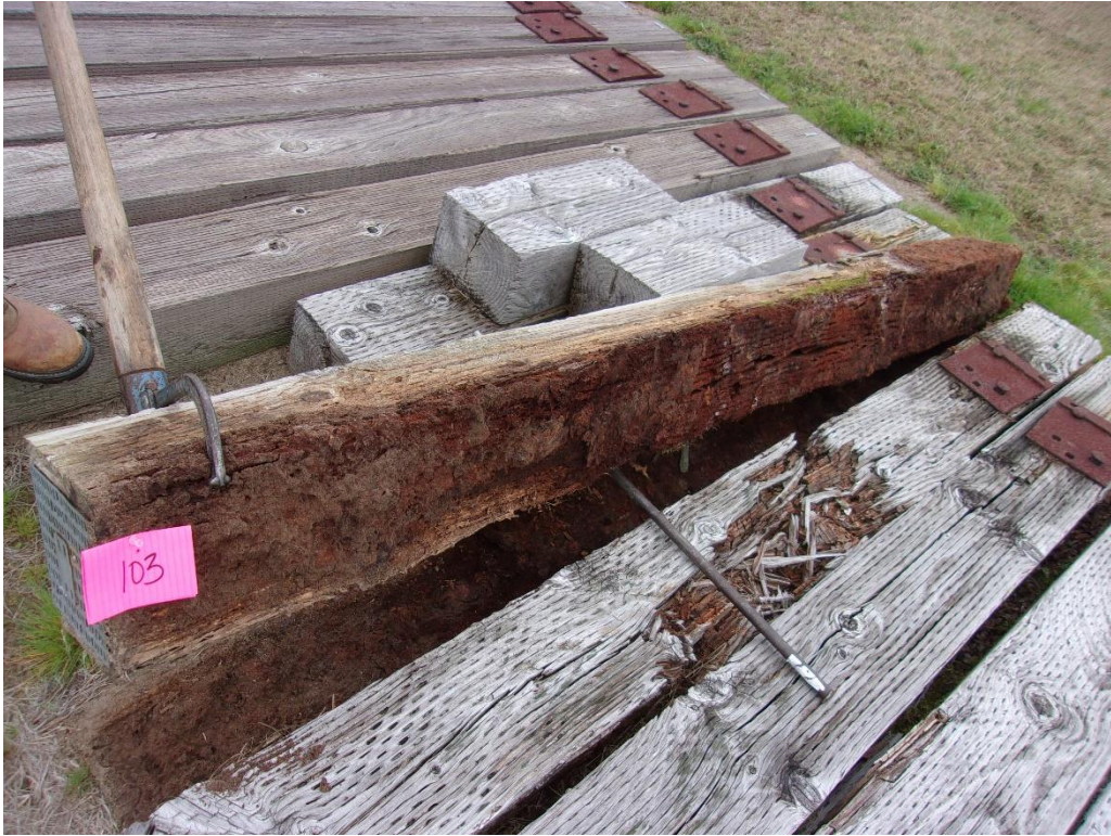
Figure 73 – Tie #103 untreated Douglas fir with decay and termite damage.
