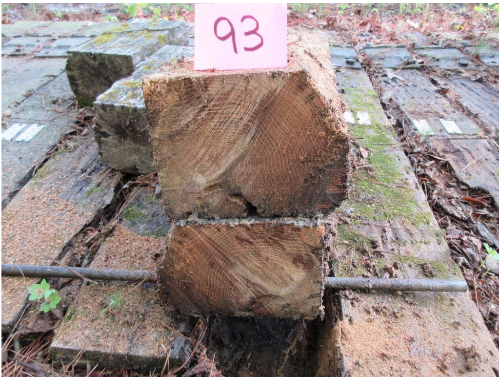
Figure 20 – Tie #93 untreated white oak with obvious decay visible.
