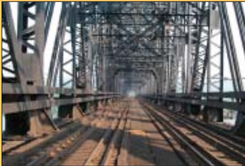
1,787 feet doesn't look all that long from this perspective, but Taubken explains it feels like more than a mile when you are in the center of it working and a 150-car train passes by at full speed. "Even a sturdy structure like this one sways and gives under those loads. It's quite a lonely feeling for a bridge crew."
